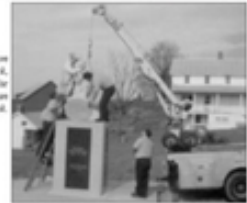
With the use of Babylon Vault's crane track, placing the 1.5-ton granite statue on its pedestal is an easier task.
